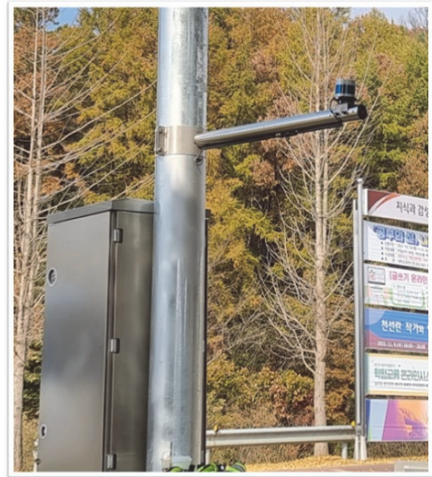
Photo 5 System installation location
